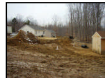
New Pump House (right) for Combined Well and Rainwater System Controls
