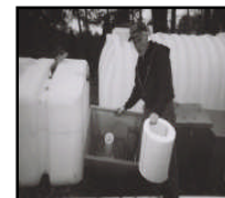
Doug Phillips Shows Some Components of the Potable Rainwater System, the Roof Washer Collection Unit Filter (in hand), and Storage Tanks (in background)
